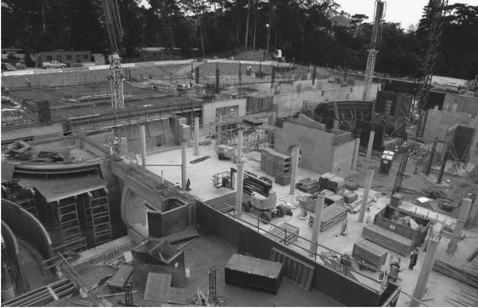
The aquarium under construction in June 2006. Everything visible is at the lower level, with the Philippine Coral Reef in the foreground, Water Planet at center. California Coast is the round window just to the right, and the beginnings of the Rainforest are at far right. Photo by Tom Hennes, courtesy of Thinc Design.
